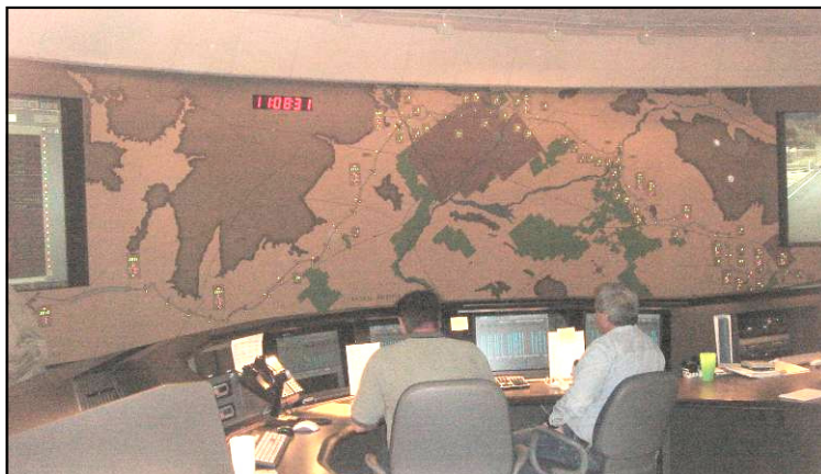
Visiting with the operators in the control room was a highlight of our recent field trip to the headquarters of the Central Arizona Project.
